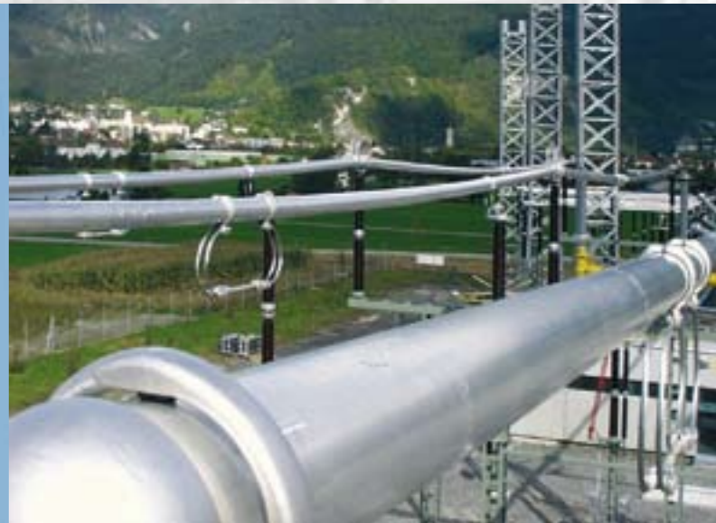
220 kV Bürs / illwerke vkw Austria
